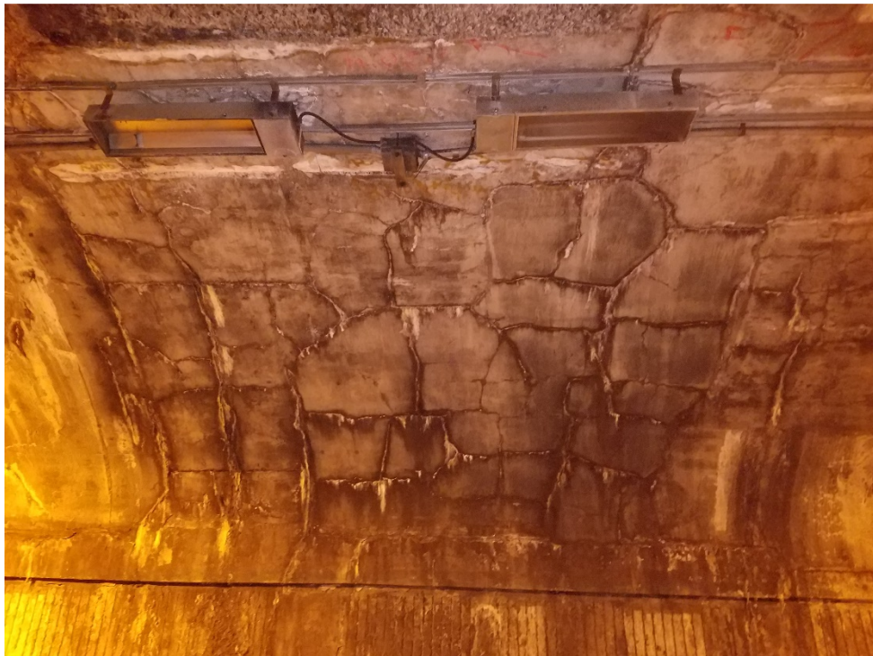
Photo 18: Inoperable tunnel lighting. Note condition of concrete tunnel liner with extensive map cracking and efflorescence.
