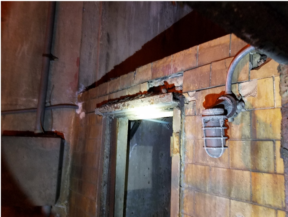
Photo 16: Lighting in control room no longer functioning.
