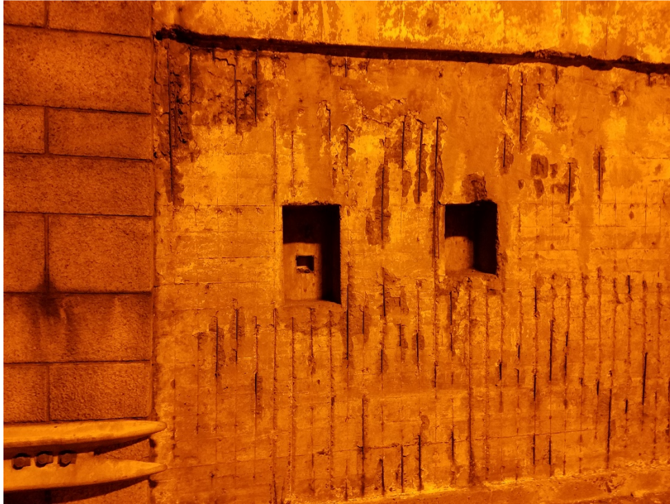
Photo 3: Remains of Telephone (Left) and Traffic Control Niche (Right) at West Portal SB Barrel. Similar arrangement at all Portals.
