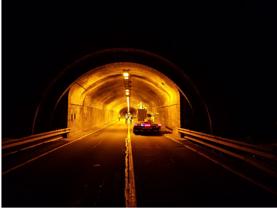
Photo 19: Lighting at tunnel portal.
