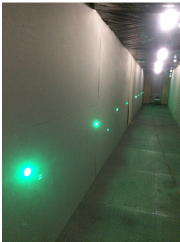
Figure 9. LED path lights in simulated tunnel.
