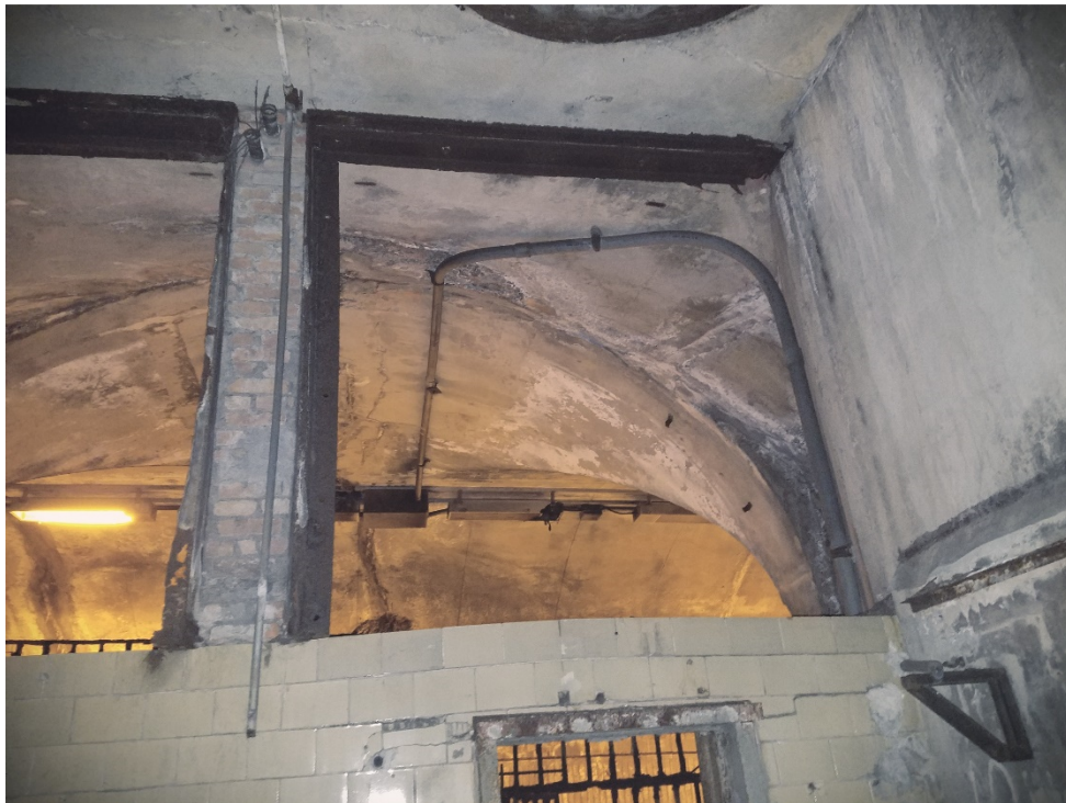
Photo 10: Dual openings for ventilation fans that have been removed.
