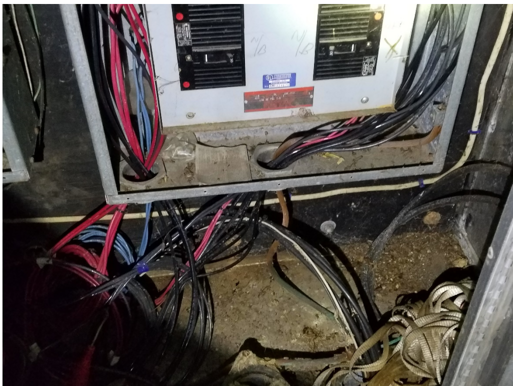
Photo 30: Daytime lighting panelboard
