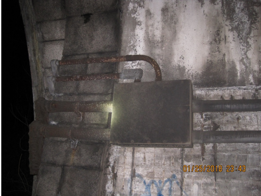
Photo 33: Additional corrosion on conduit and conduit bodies.
