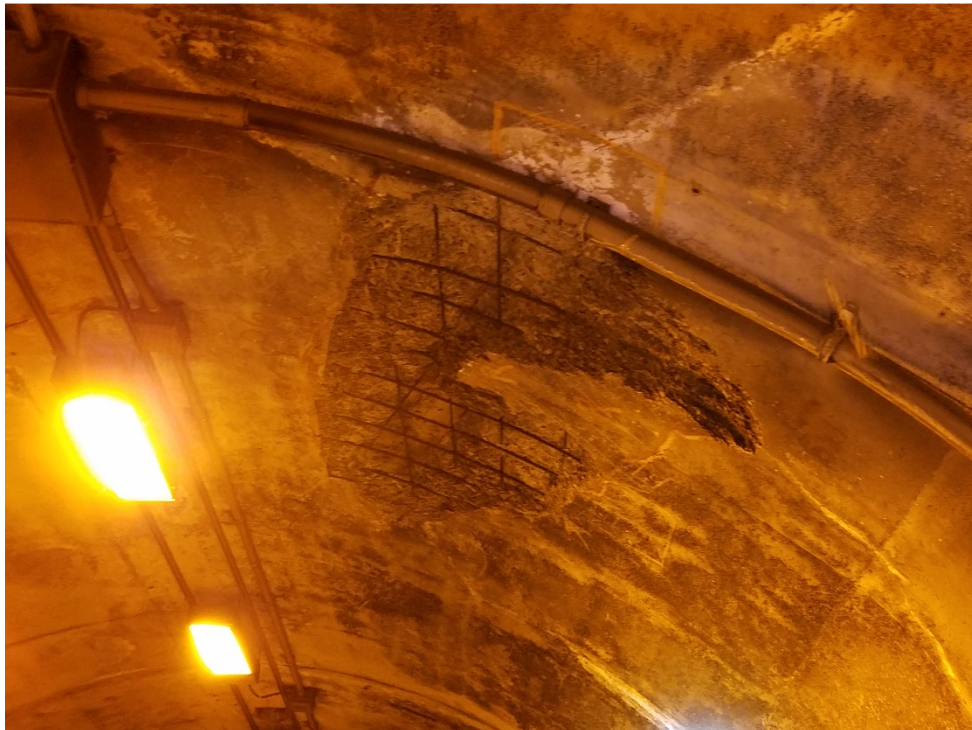
Photo 12: Existing concrete tunnel liner. Note the deterioration and exposed rebar, all conditions that could affect the fire resistance of the existing concrete tunnel liner.
