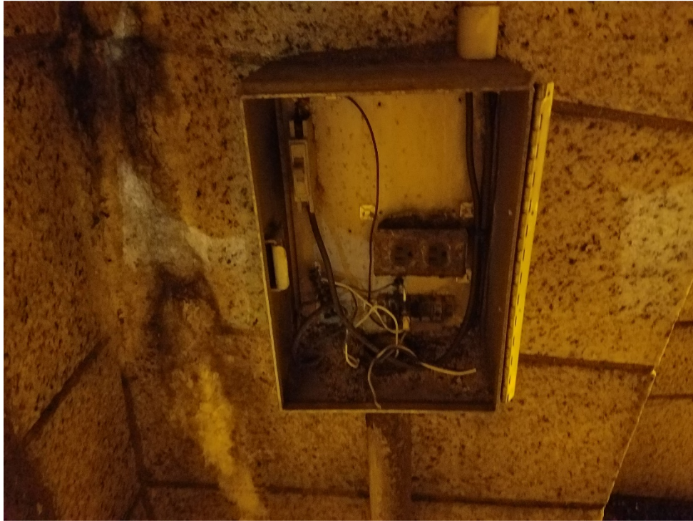
Photo 13: Abandoned Electrical Junction Box with exposed wiring.
