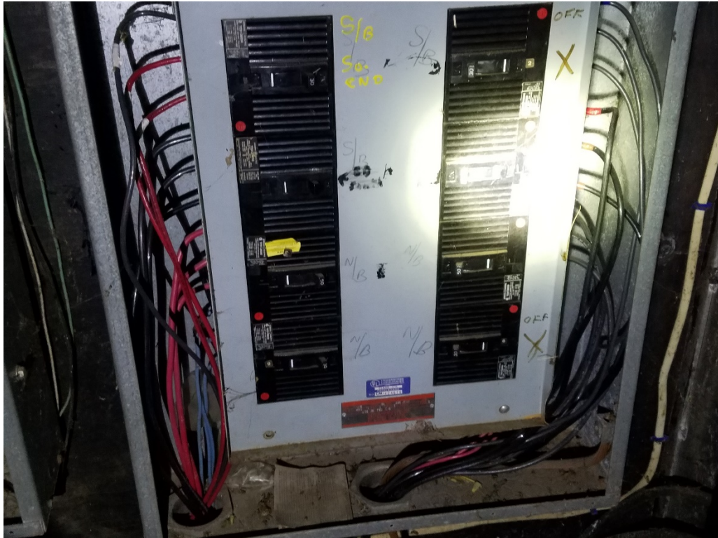
Photo 29: Daytime lighting panelboard
