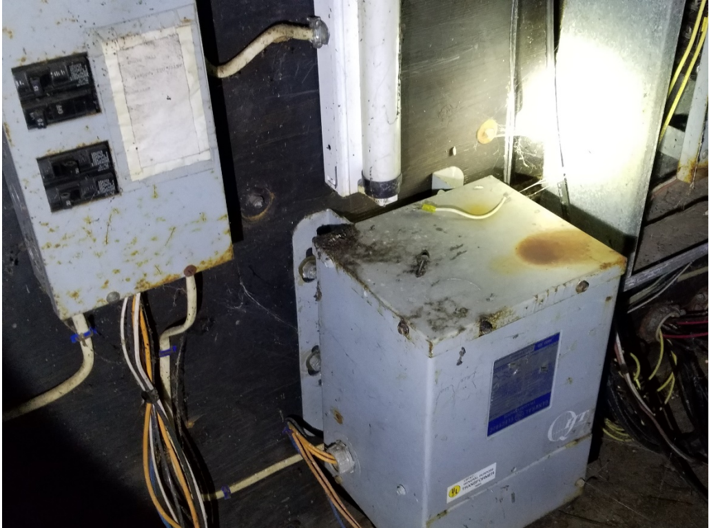
Photo 27: 120V Panelboard (Left), 480-120/240V transformer (Right)
