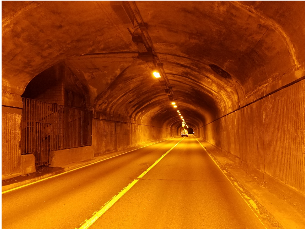
Photo 5: Existing NB Barrel Cross Section with 2'-6" safety curbs and gated entrance to abandoned control room. Also note inoperable tunnel lights in ceiling.
