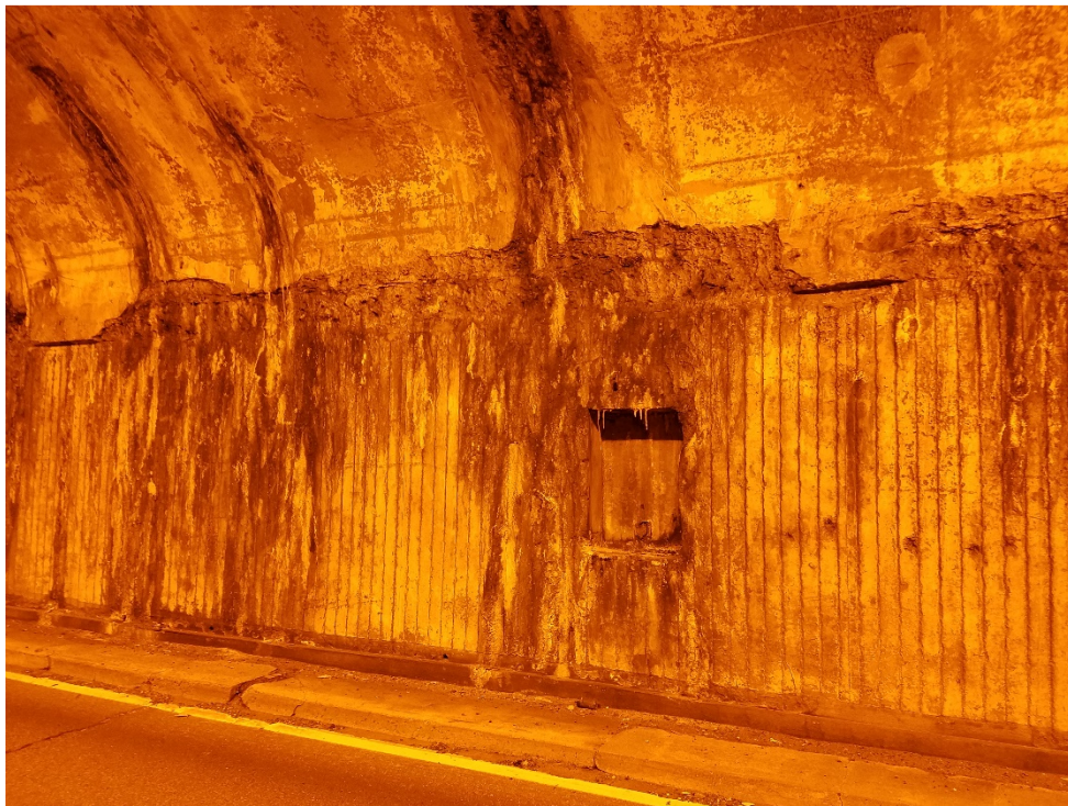
Photo 4: Remains of Fire Extinguisher Niche. Note deterioration in tunnel liner wall.
