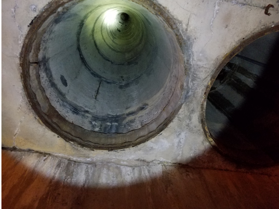
Photo 11: Existing 6'-0" diameter ventilation shaft. Note the evidence of leakage at joints in shaft.
