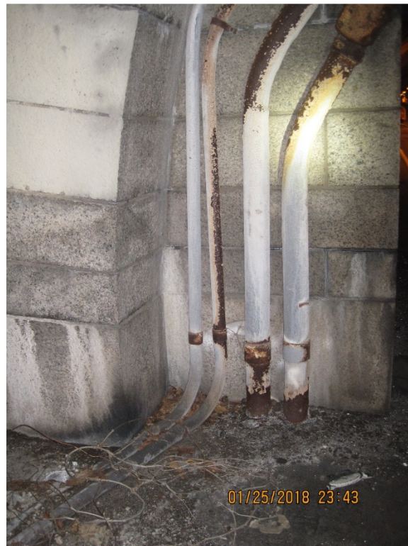
Photo 32: Corroded conduits containing lighting and Wintergreen Avenue electrical service wiring.
