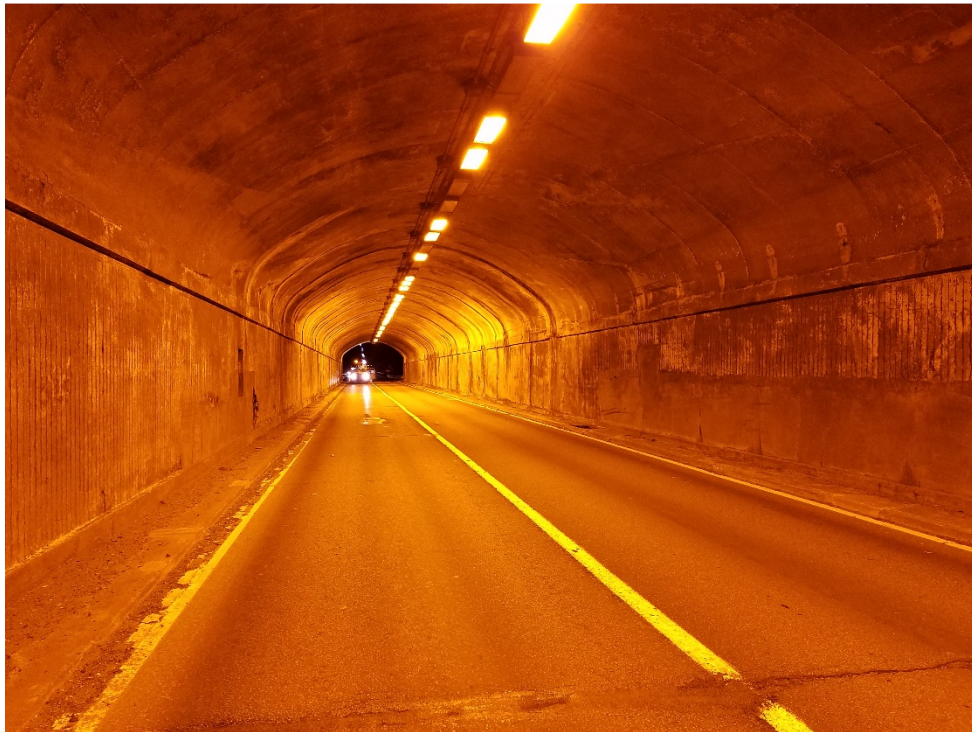
Photo 20: Tunnel lighting with random luminaires no longer functioning.
