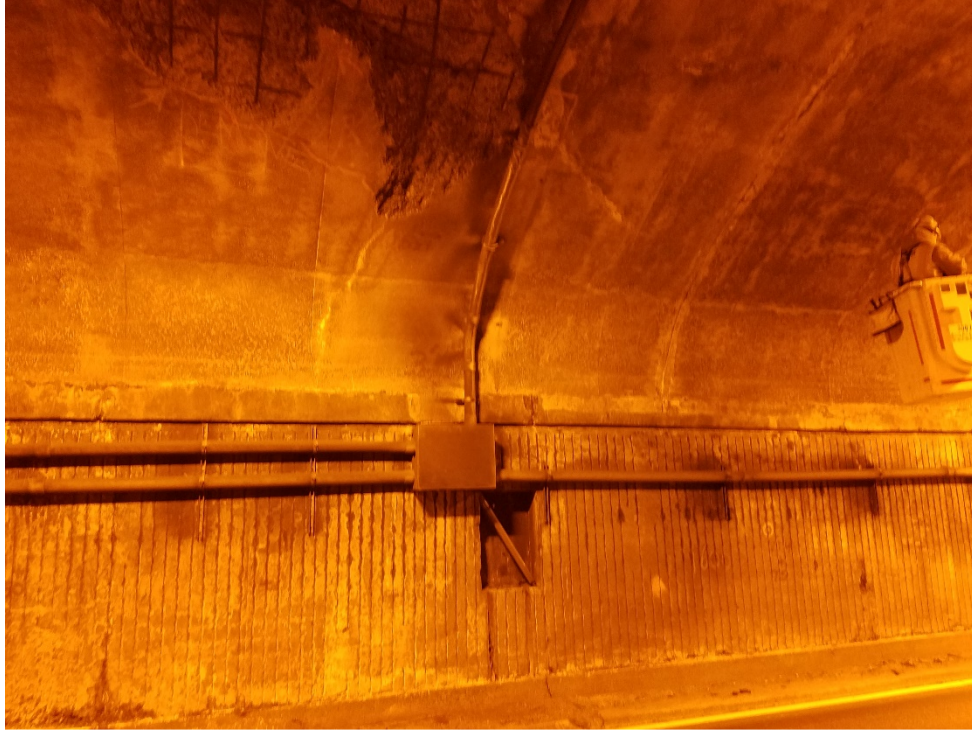
Photo 17: Conduit in SB Barrel at tunnel centerline with junction box and a run of conduit mounted to ceiling going to the lighting system.
