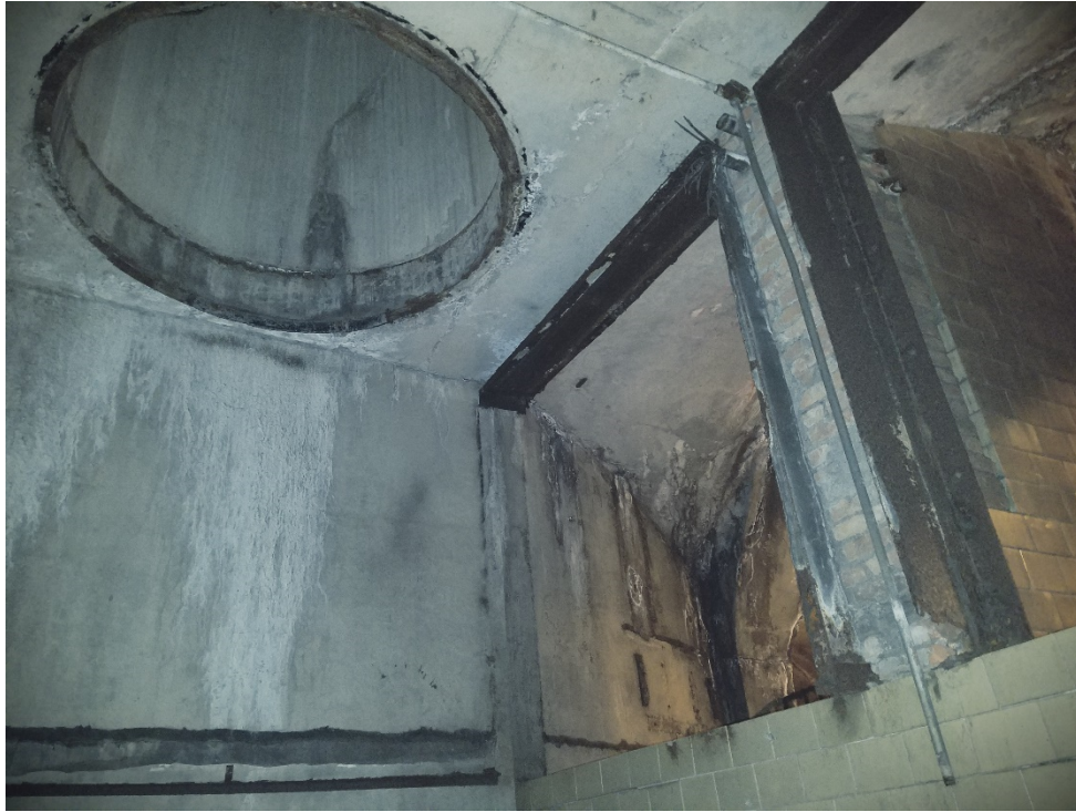
Photo 9: Control room showing rectangular opening for ventilation fans and 6'0" diameter ventilation shafts leading to ventilation building at top of West Rock Ridge.
