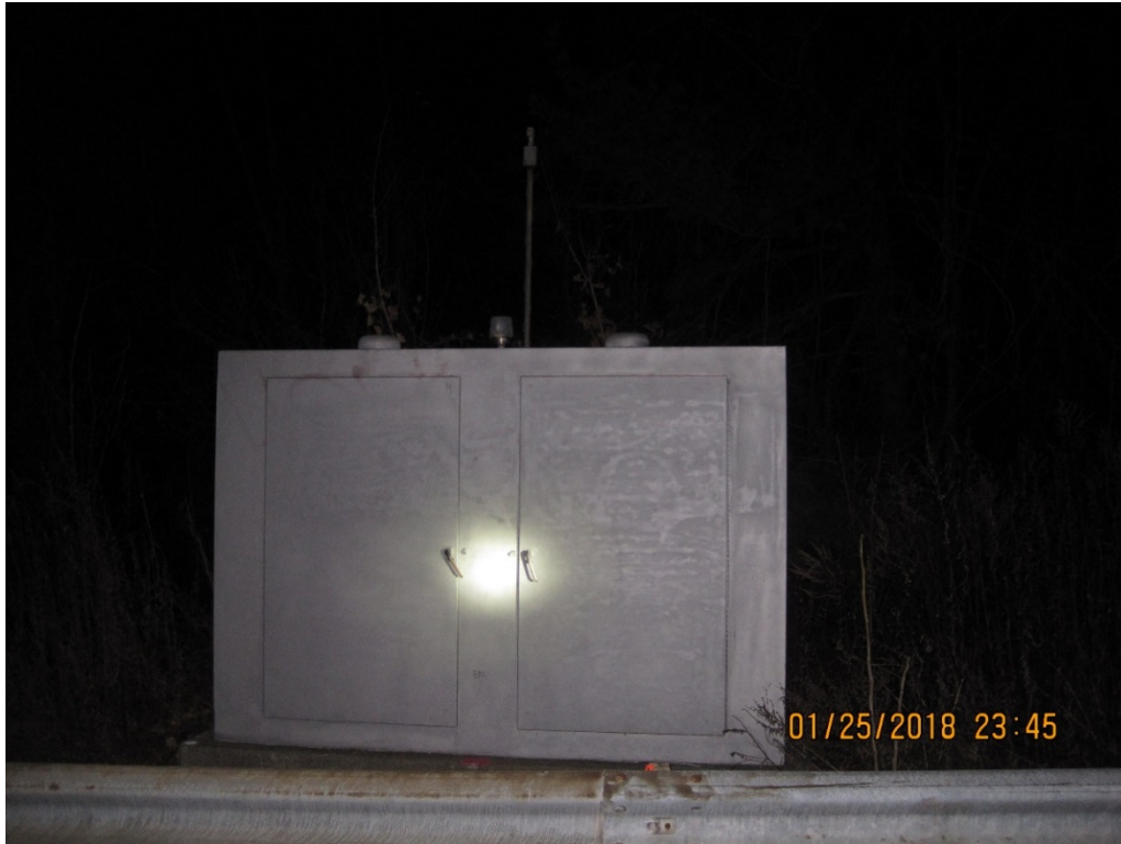
Photo 31: Electrical distribution pedestal cabinet
