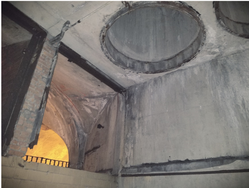
Photo 8: Control room showing rectangular opening for ventilation fans and 6'0" diameter ventilation shafts leading to ventilation building at top of West Rock Ridge.
