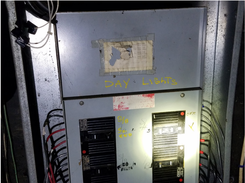
Photo 28: Daytime lighting panelboard
