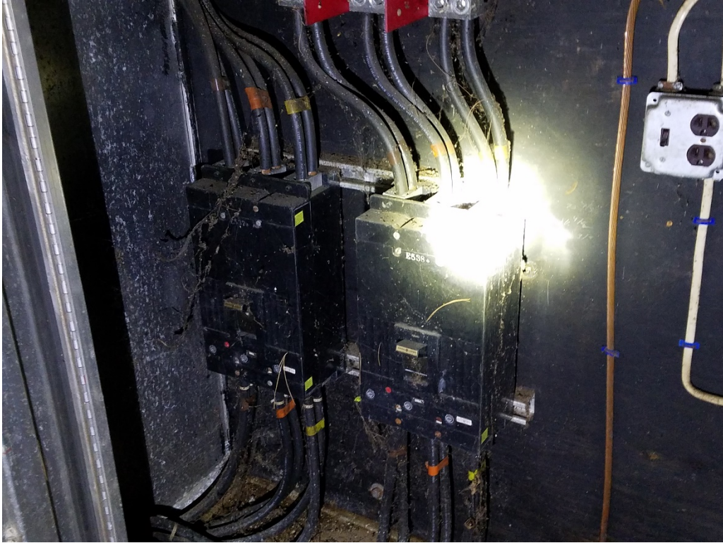
Photo 25: 500A main circuit breakers for the two utility services
