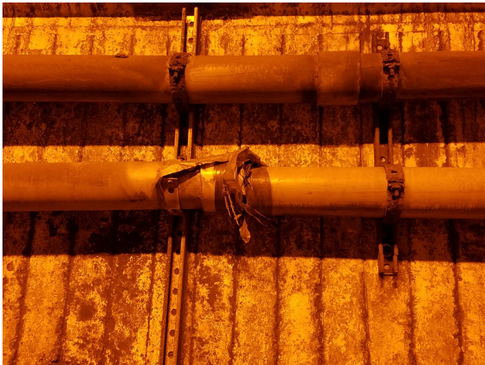
Photo 14: Existing PVC Conduit with duct tape repairing damage to the conduit.
