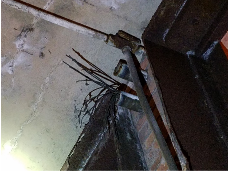
Photo 15: Abandoned conduit with exposed wiring in control room.
