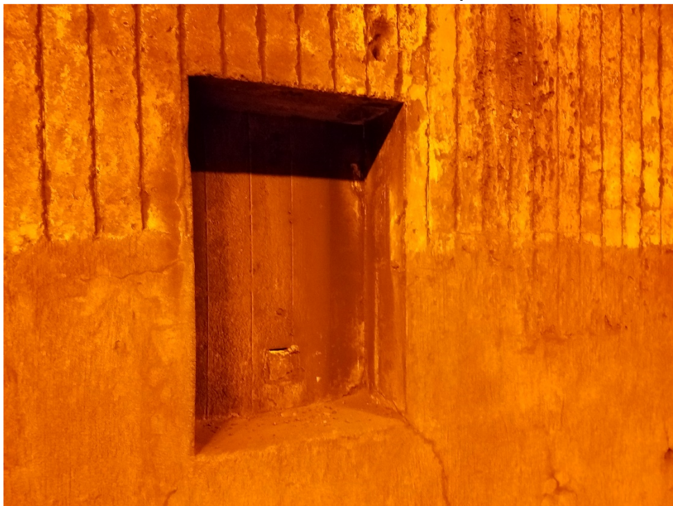
Photo 2: Remains of Fire Extinguisher Niche. Fire Extinguisher has been removed.
